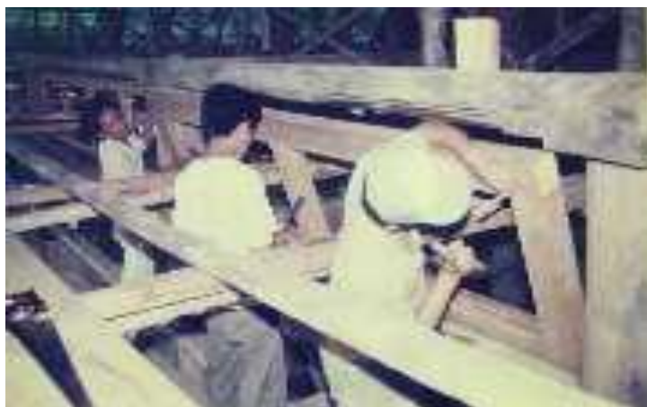
Figure 1. Photograph of the Installation of Wooden Wall Beams and Ventilation Source: Cultural Heritage Preservation Agency (BPCB) East Java
